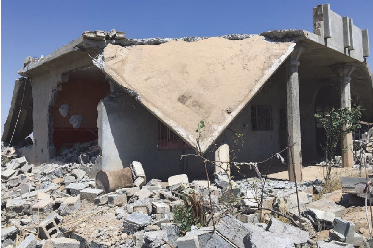
House destroyed with a bulldozer in Qarah Tappah May 2016. © 2016 Human Rights Watch
