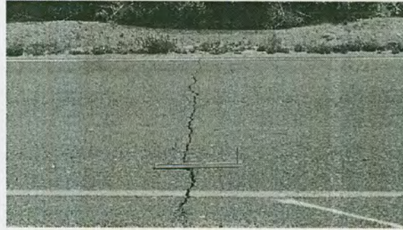
Figure (2-4) Thermal Cracking of Asphalt Paved Road (Fwa, 2006)
