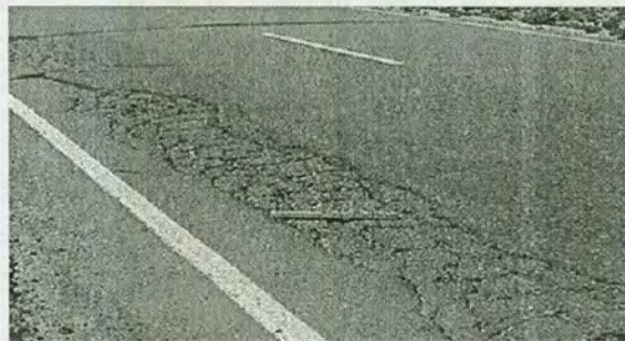
Figure (2-5) Fatigue Cracking (Fwa, 2006)
