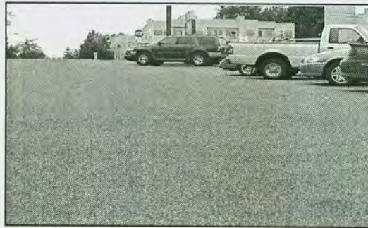
Figure (2-3) Corrugated Distress ( www.pavementinteractive.org ).
