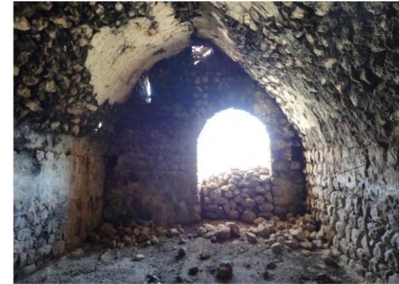
Khaana Ezid interior, 2011 – The interior is dominated by parallel vaults. The masonry shows in small reference surfaces a homogeneous plasterwork on walls and ceilings.
