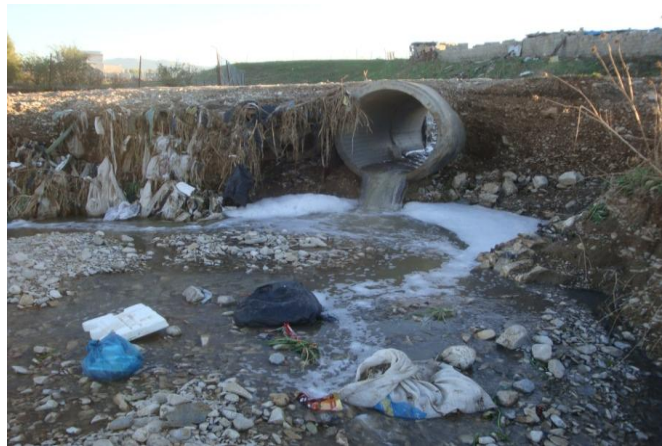
B: Sewage effluent boxes at north west-Halabja City
