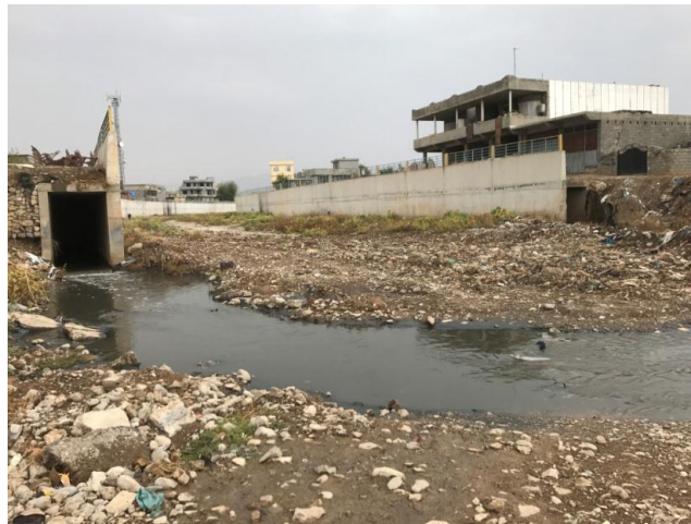
C: Sewage effluent boxes at NW of SaidSadiq District
