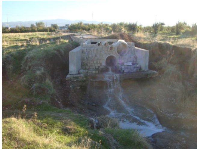
A: Sewage effluent boxes at south east -Halabja City
