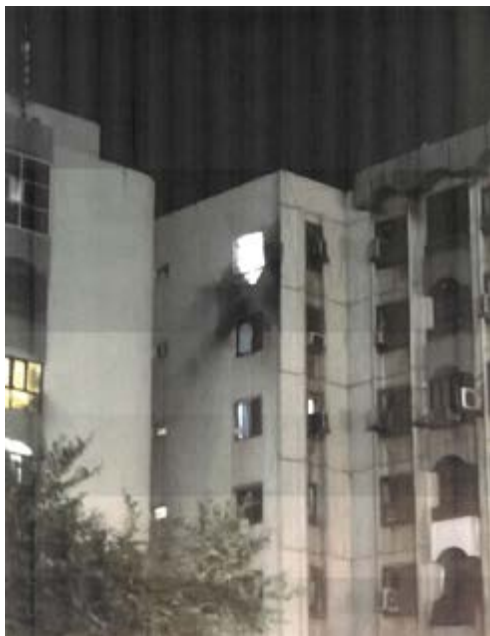
Damage from a December 20 rocket attack on U.S. Embassy buildings in Baghdad. (DoD photo)
