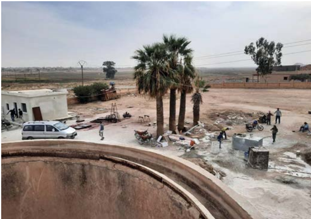
Rehabilitation of Shaddadi Desalination Plant will provide a sustainable water supply to an estimated 9,000 beneficiaries in al-Shaddadi. (USAID photo)
