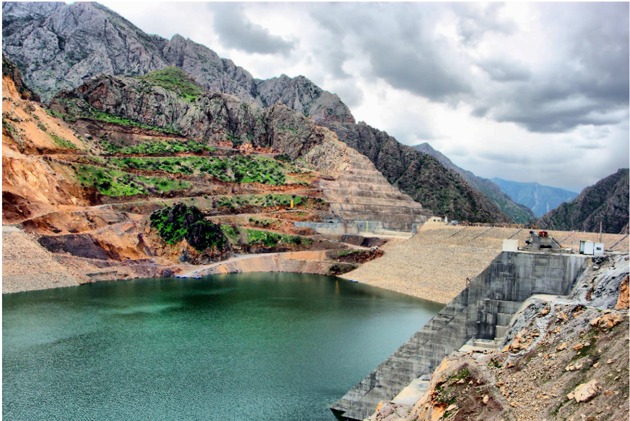
Figure 1. The Daryan Dam under construction on the Sirwan River in Iranian Kurdistan (Arash Bahrammirzaee, 2016)
