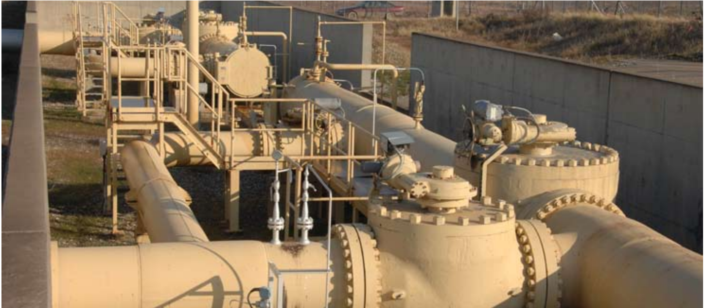
Existing export line and fiscal metering station at tie-in area in Fishkhabour
