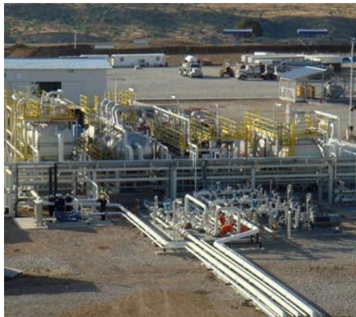
Central Processing Facility
