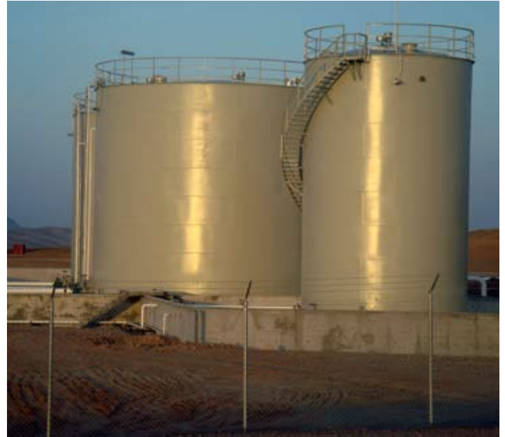
Tawke CPF crude storage tanks
