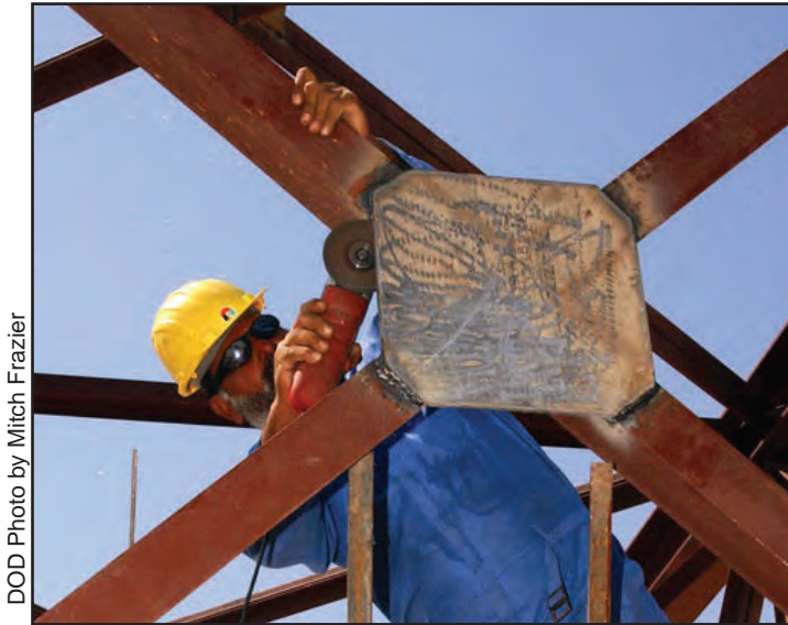
Figure 133. An Iraqi laborer grinds a plate on a metal support structure at a military training base in eastern Iraq. The structure supported a water storage tank that will soon supply the base with clean water.
