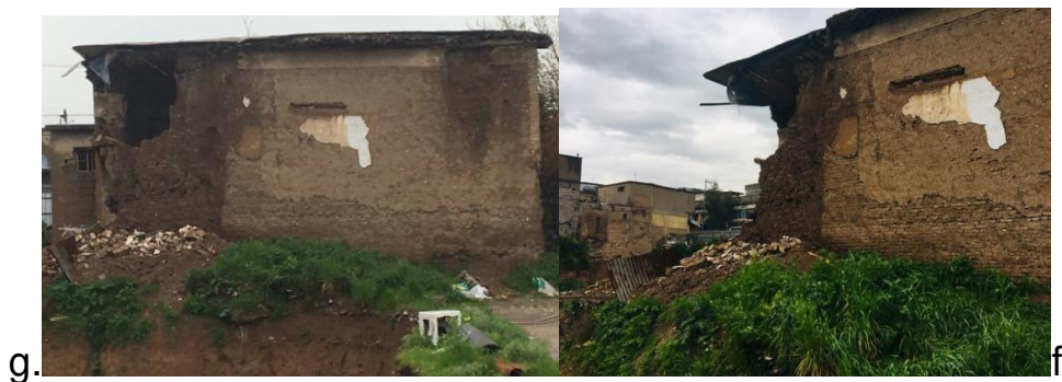
Fig.8.f-g. The Ahmed Qopch building, its western corner and its façade collapsed due to the earthquake and the heavy storm raining of the early spring 2019. (Photo by the author in April 2019).
