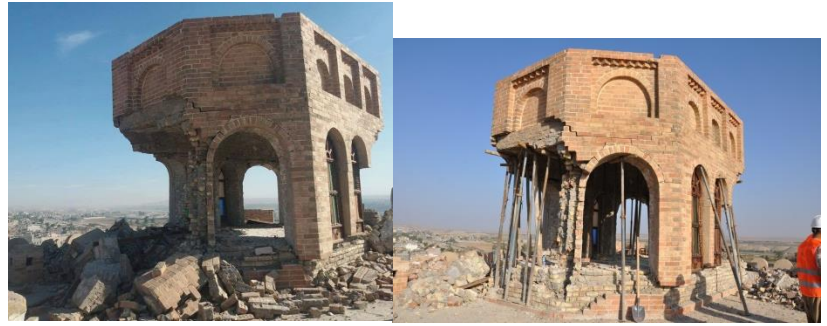
Fig. 6.a. The cracks on the wall of the attic of the castle, caused by an earthquake in 2013. ((Photo by Nawzad Latif, Archive of the Directorate of Antiquities of Garmian).
