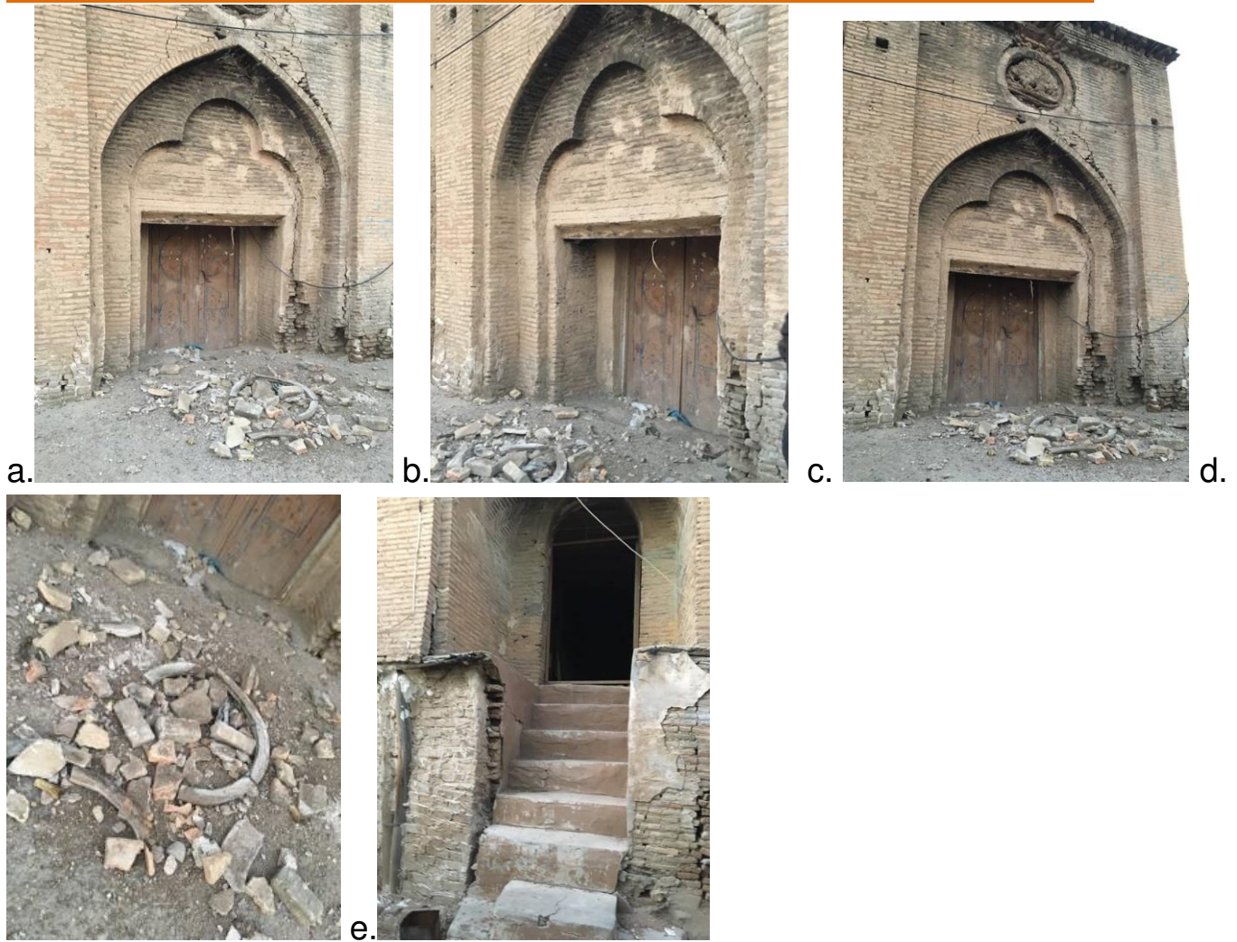
Fig.8. a-e. The earthquake made cracks on the sides of the gate and the fallen ornaments from the façade of the Ahmed Qopcha heritage building in Sulaimani (photos by the author November 2017).
