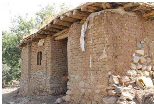
Fig. 8 A: A mud brick house with flat roof in Sidekan. The roof is built from reeds and wooden spars overlaid with leaves and mud. (Photo by author).
