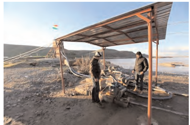
Iraqi Kurds stand near pipes that feed diesel from a pumping station in Iraqi Kurdistan to Syria on the Iraqi bank of the river Tigris at the Iraqi-Syrian border near the Dohuk province, February 2, 2013. (REUTERS/Azad Lashkari)
